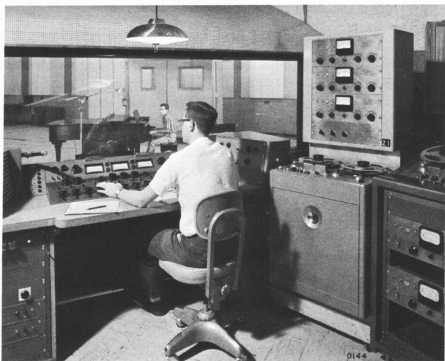
Magnetic equipment in the recording industry. Ampex Model 300-3 installed at United Recording Studios, Hollywood.
